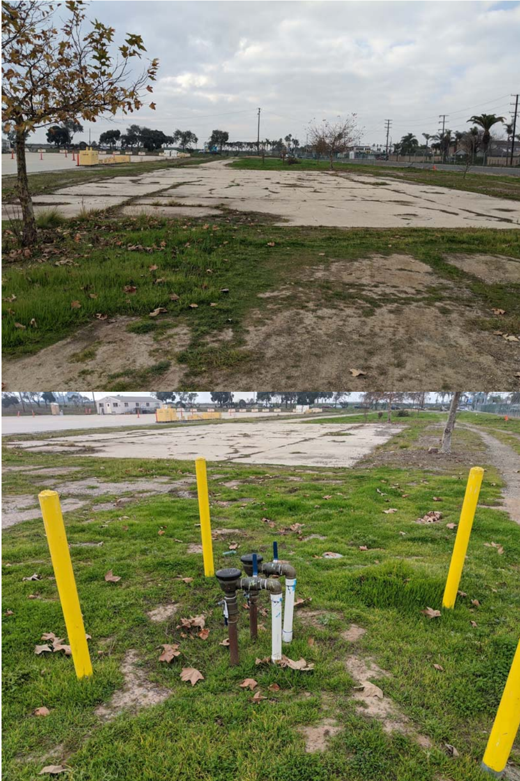
Concrete pads on west section of subject property looking south (top) and irrigation line at same location (bottom)
