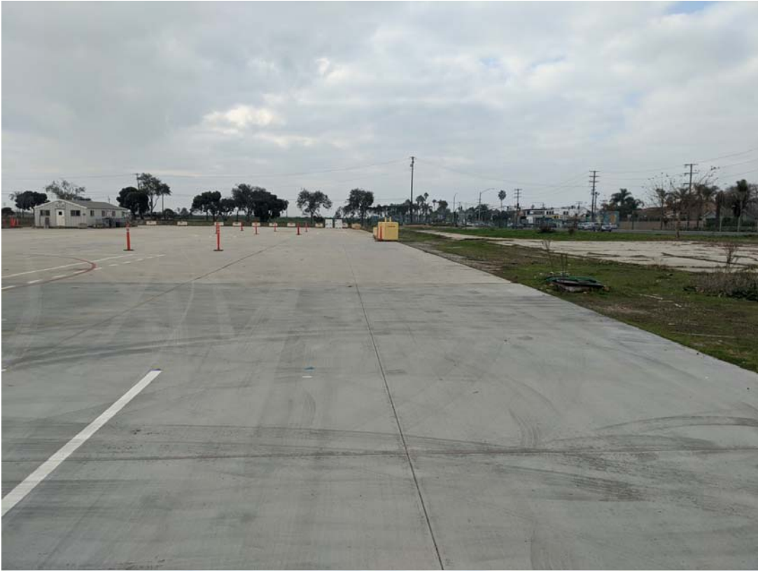
Concrete pad (top) and looking west towards pre-fab structure on concrete pad (bottom)
